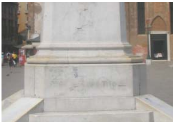
Figure 13: Vandalism to a monument
