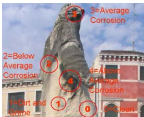
Figure 22: Severity Condition Assessment
