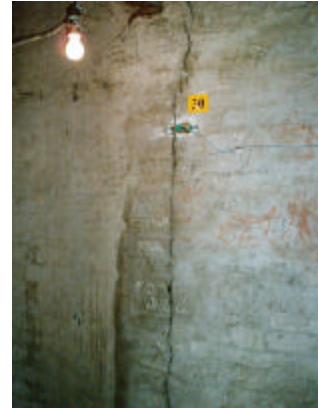
Figure 22- Crack and Strain Gage
