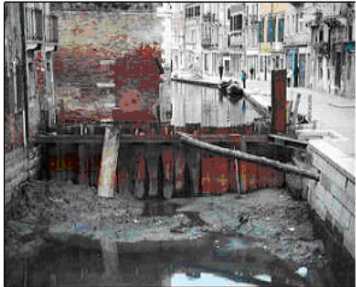
Figure 4: Canal Wall Damage and Repair Work
