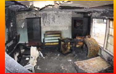
Post fire damage
